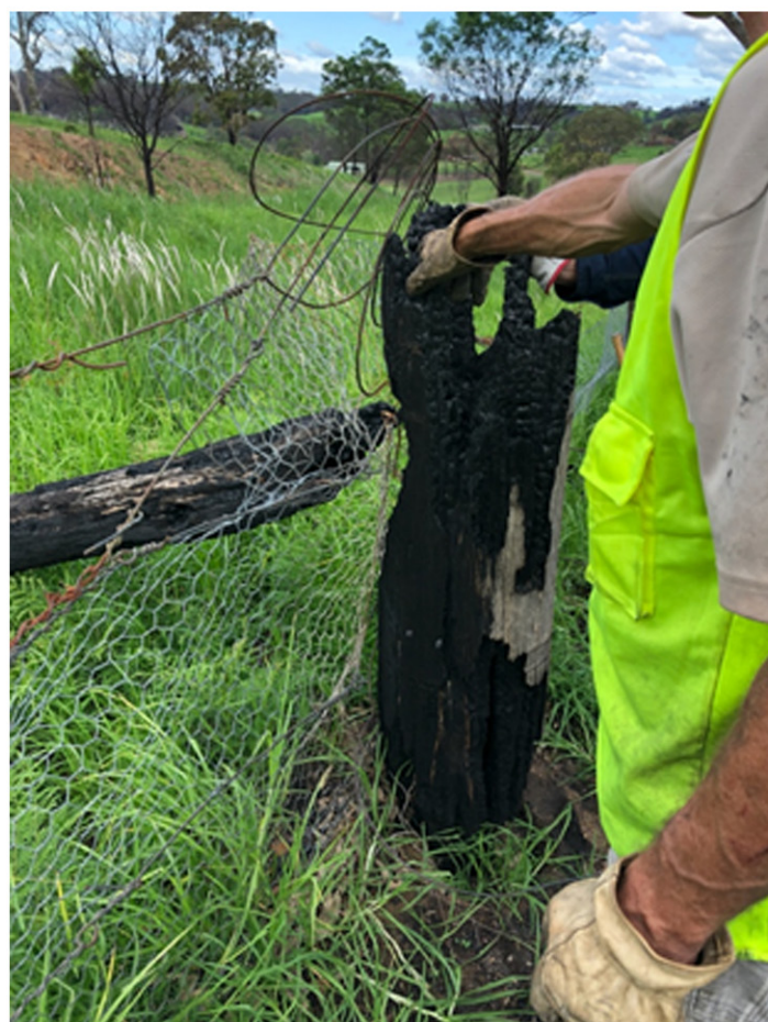
One of the main posts, burned off at the ground. Cattle can simply push against the fence and walk over it.
